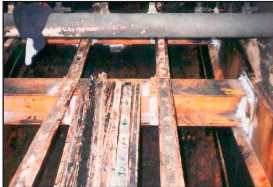
Damaged coal screen
